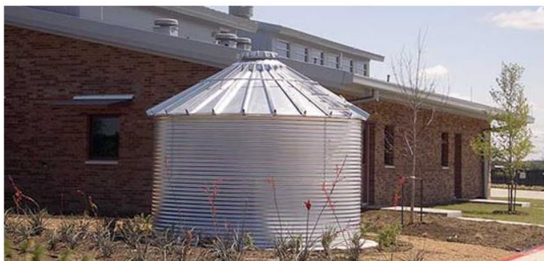
Photo: "IWS - watercache.com"; 5600 gallon commercial rainwater collection system for LEED Gold rated fire station in Denton, Texas. Rainwater is used to irrigate native plant landscaping around the station.
